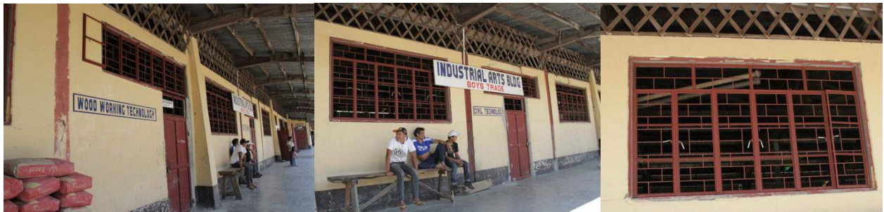
The wooden doors and windows of the Marikina type Industrial Arts Building were replaced into iron grills
