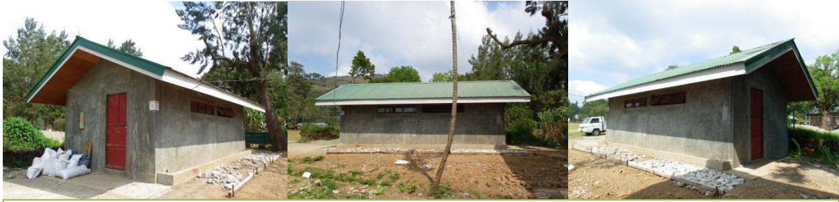
Construction of BSU SLS comfort rooms replacing old structures to serve high school students
