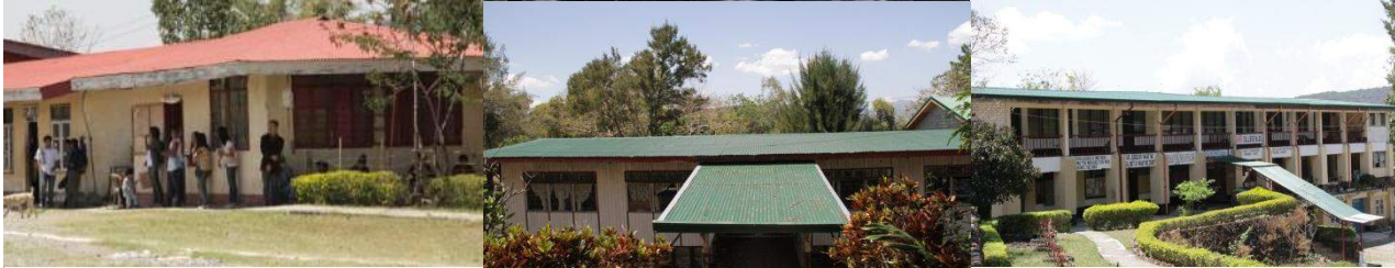
The roofs of the 13 buildings including the dormitory and cottage were repaired and painted
