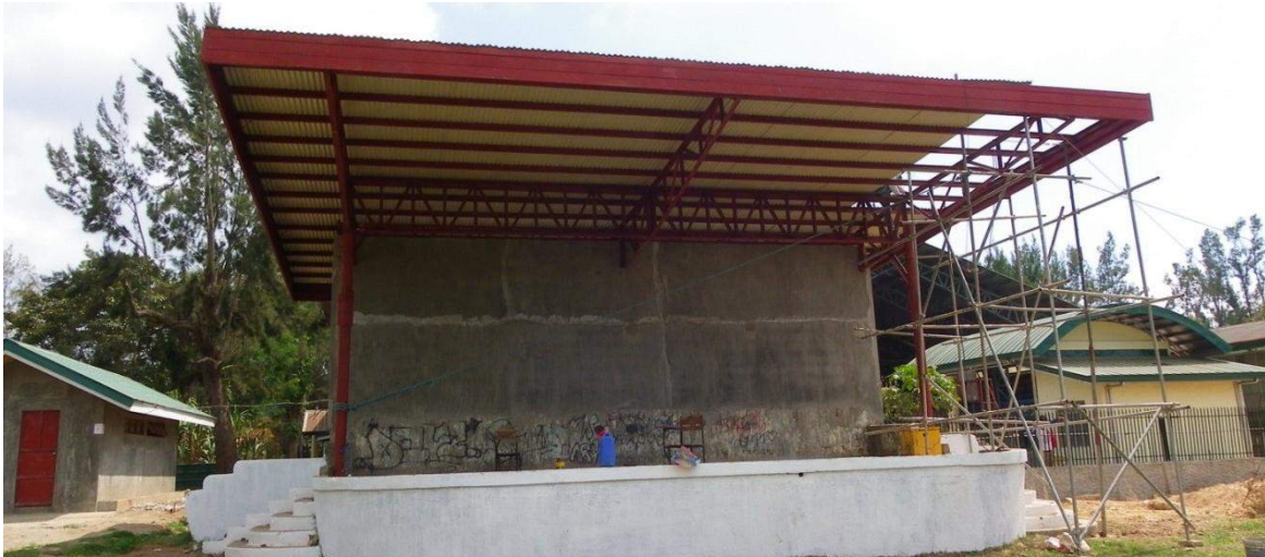
The Citizenship Advancement Training (CAT) stage and armory was restored/renovated after decades of neglect
