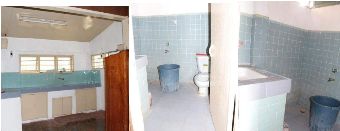
The two comfort rooms and the kitchen of the Executive Dean's Cottage at Bokod campus were repaired
