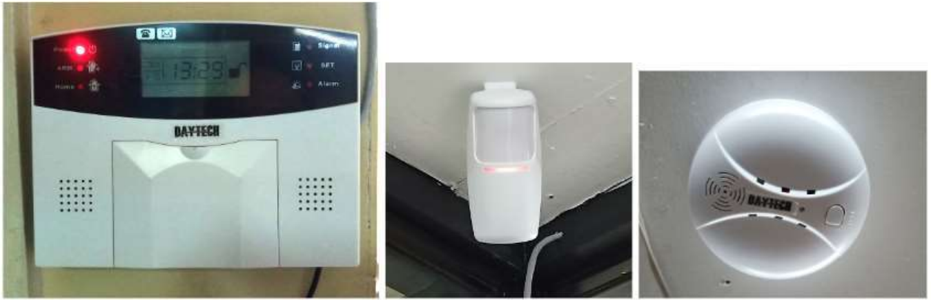
Figure 1. Alarm System at ICT-NOC
